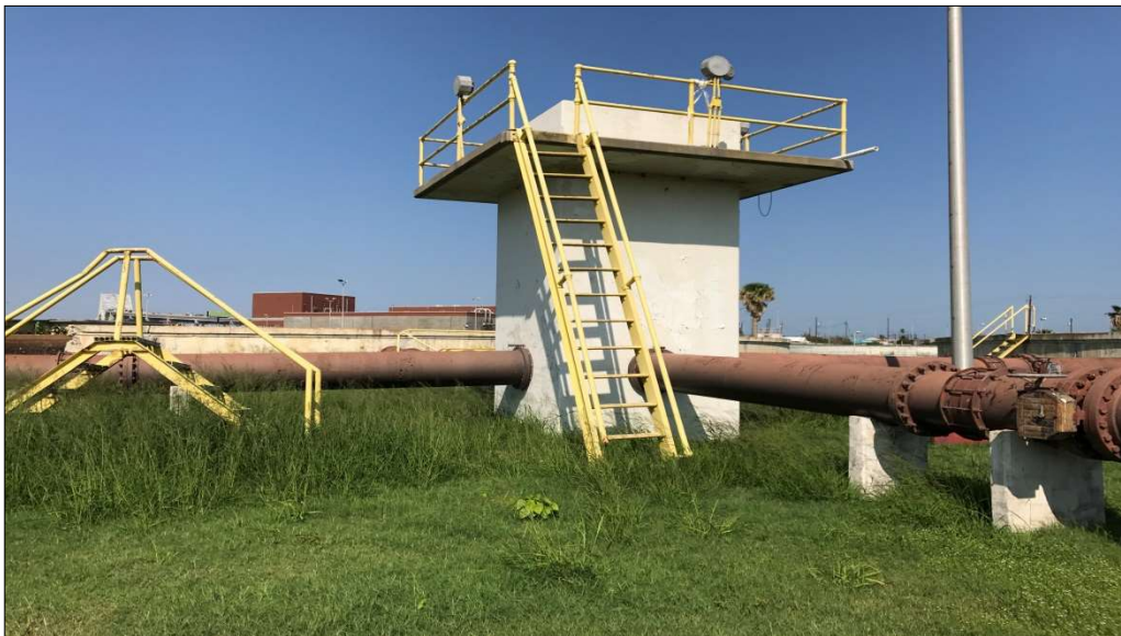
Photograph 9: Photograph of the Decommissioned Modified Distribution Box
