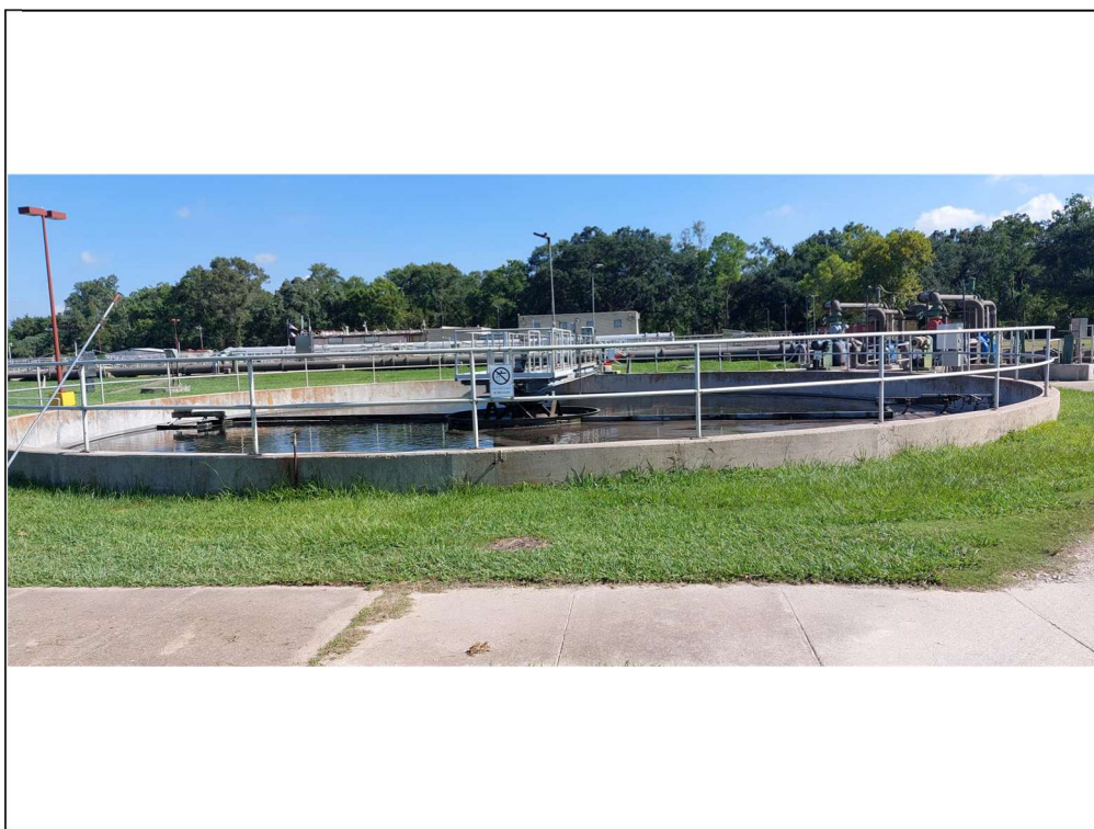
Photo 6 – Clarifier 3 and RAS Pump Station
