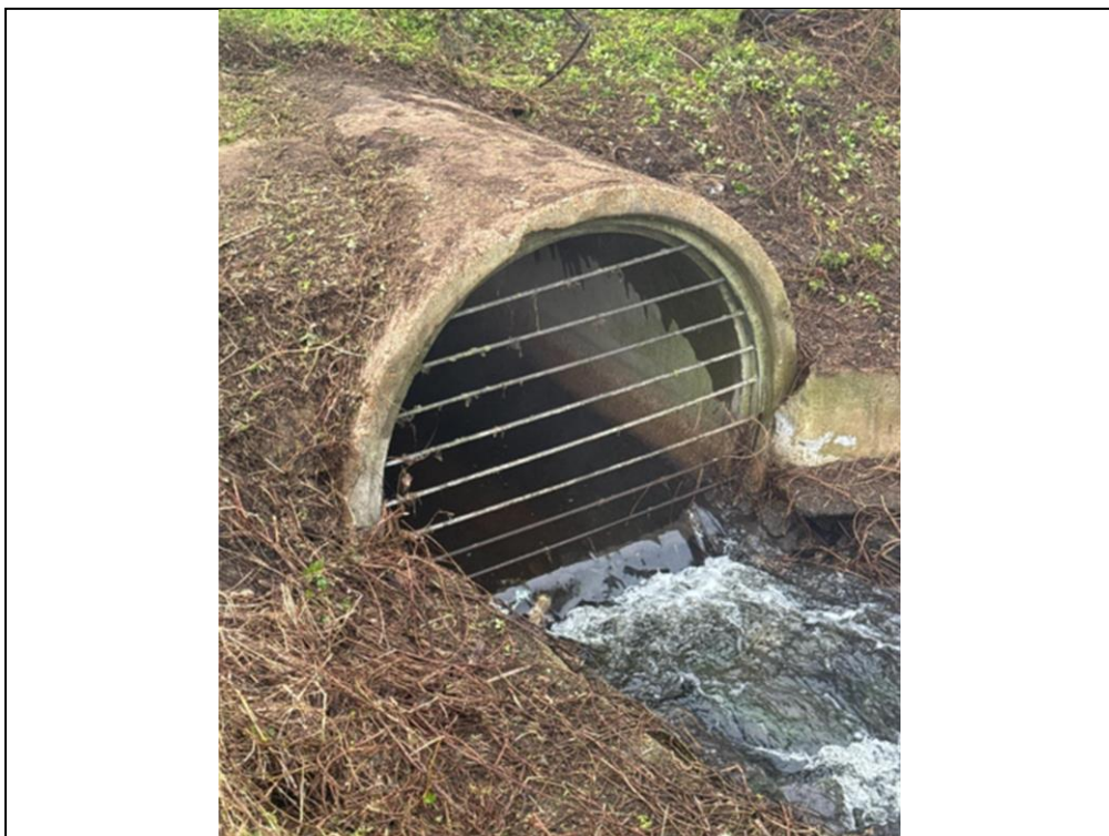
Photo 3 – Robert T Savely Outfall 001 Entering Horse Pen Bayou
