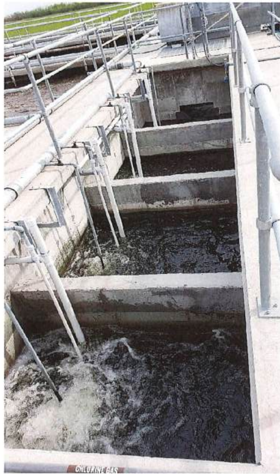
Image 14: Chlorine Contact Chamber 2
