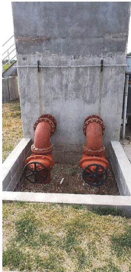
Image 2: Gate Valves on Headworks
