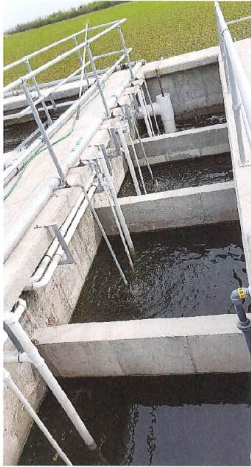
Image 15: Chlorine Contact Chamber 1
