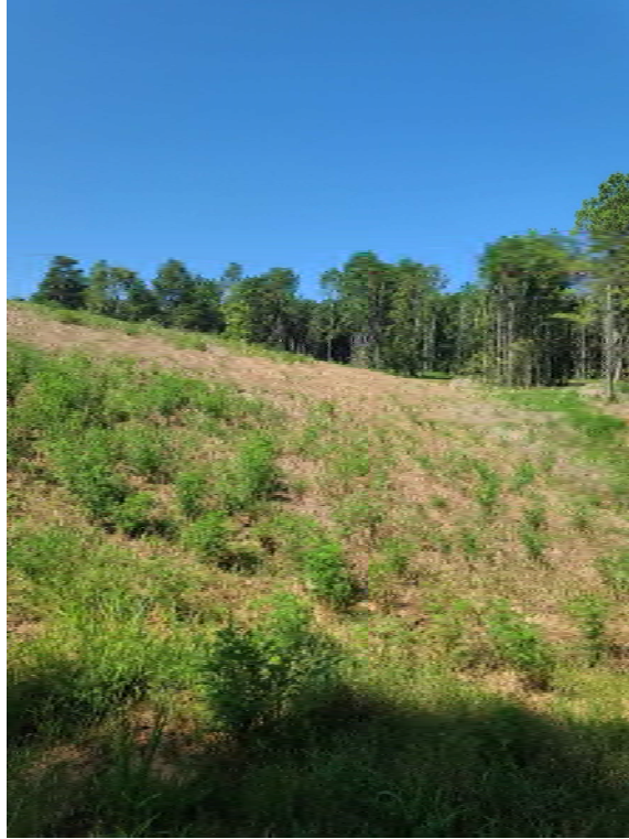
Photo 5. Viewing the stabilized dam with vegetation on the northeastern part of the property facing west.
