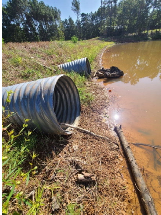
Photo 1. Viewing culverts on the north side of the impoundment on the northern part of the property from the west facing east.
