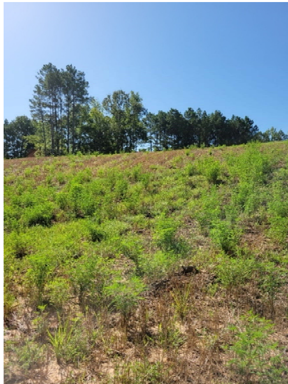
Photo 4. Viewing the stabilized dam with vegetation on the northern part of the property facing southeast.
