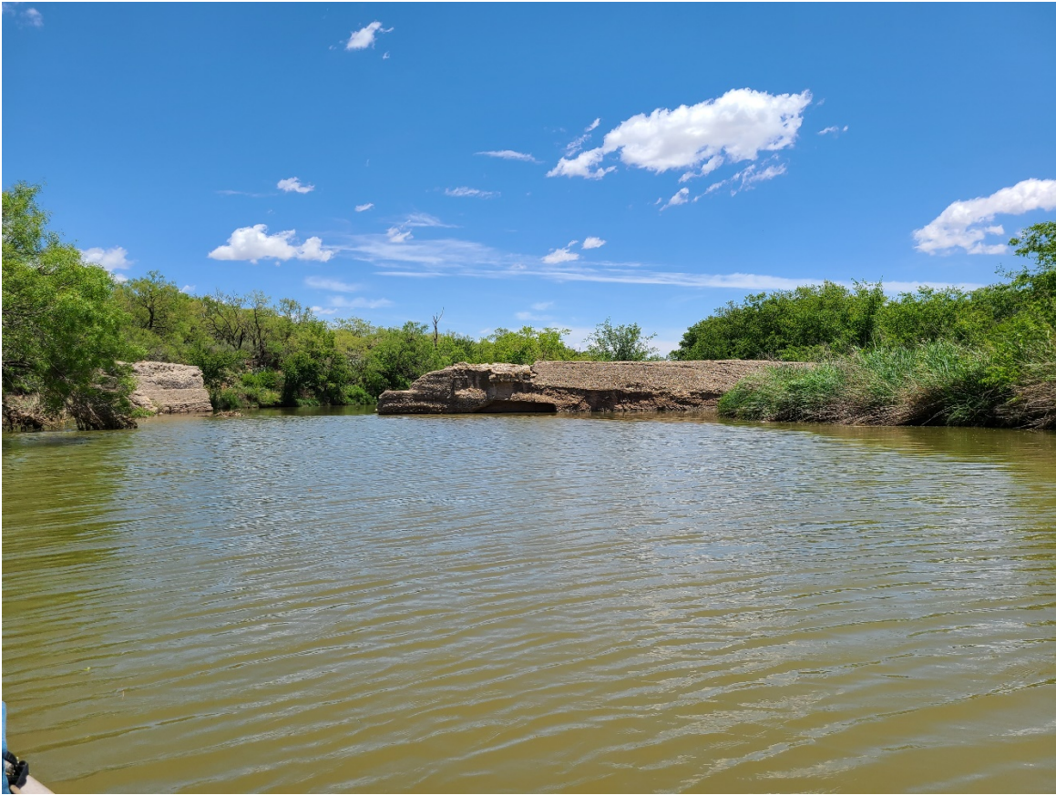
Photo 5 – Failed Dam Structure within Conveyance Reach
