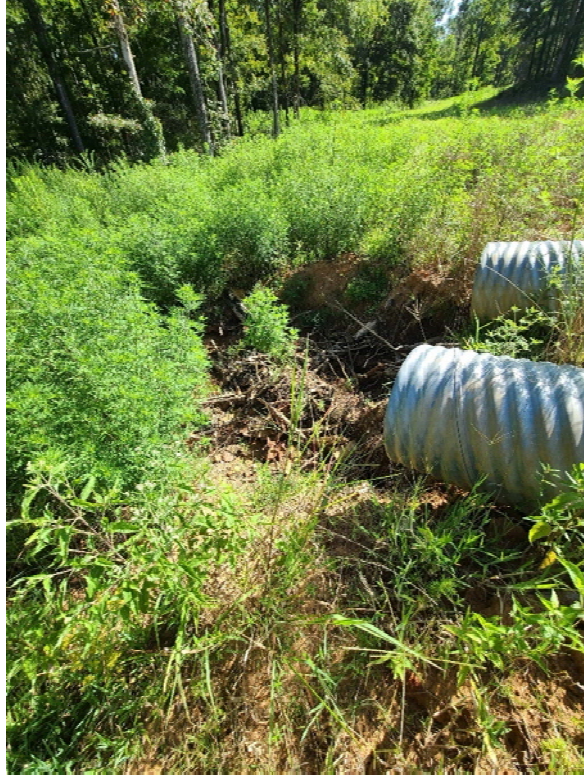
Photo 3. Viewing the culverts on the north (downstream) side of the dam on the northern part of the property facing east.
