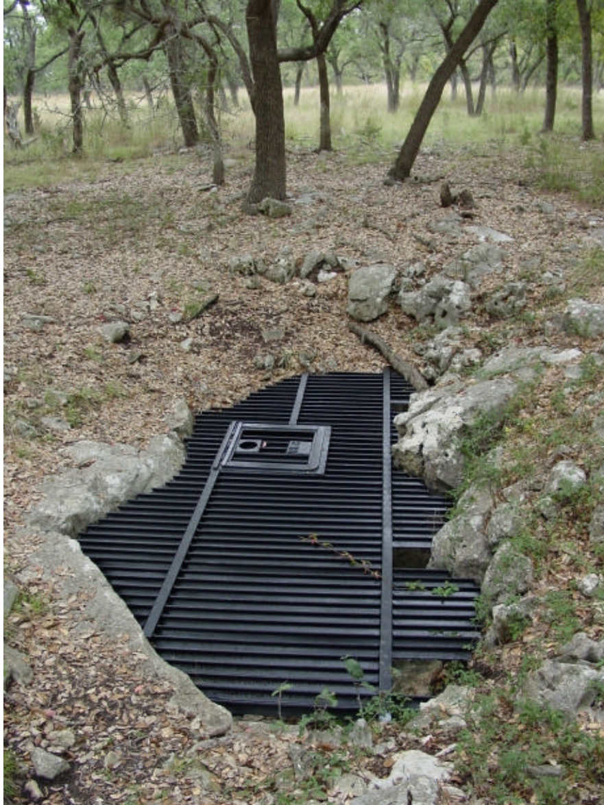
Figure 5-1 Typical Cave Gate with Secure Entrance (Mike Warton, PBS&J)
