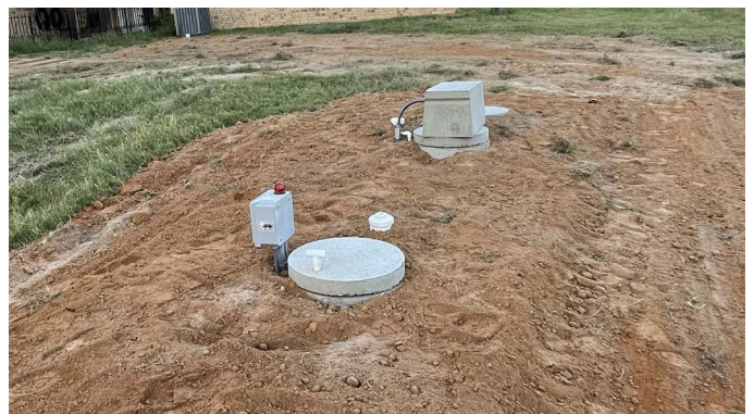
FIGURE 2.2 New septic system installed with proper sloping to prevent standing water from damaging pump (Photo by Eddie Sifuentes, CL Septic)
