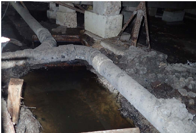
FIGURE 2.1 Pooling wastewater above septic tank in the Tres Palacios Creek watershed (Photo by Ryan Gerlich, Texas A&M Agrilife Extension Service)
