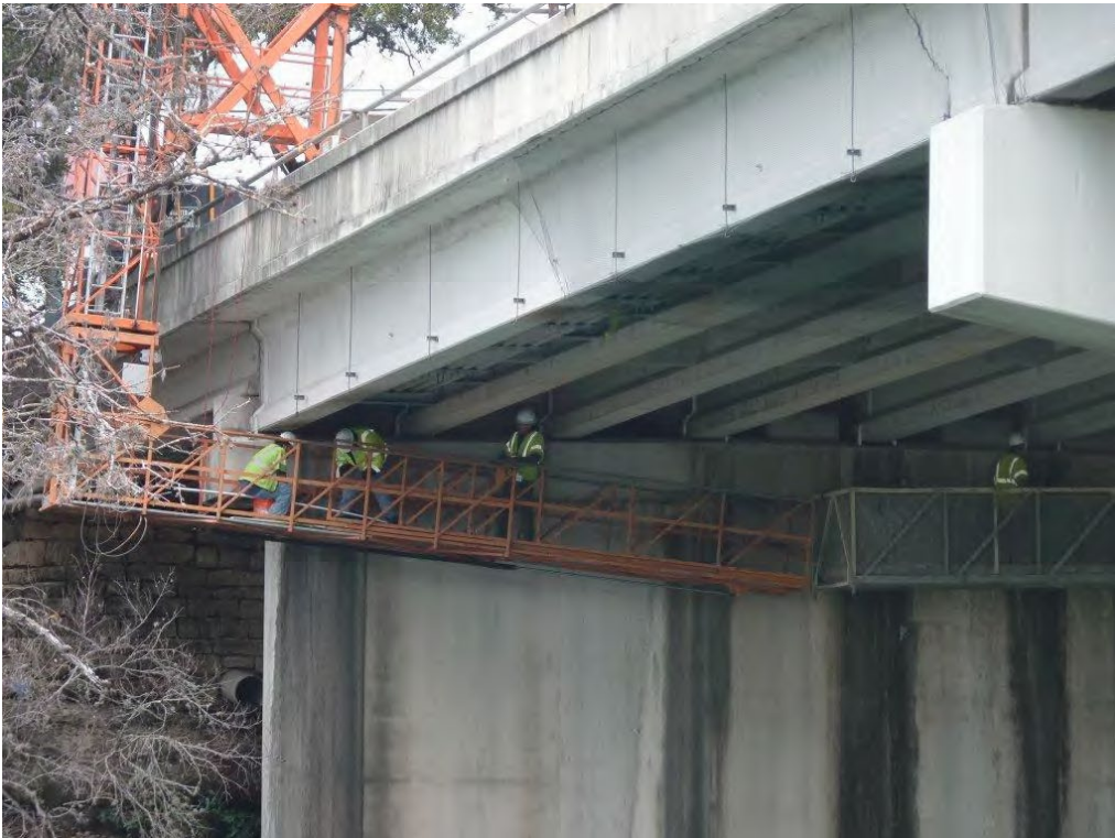
Figure 13. Netting installation taking place on span of Hwy 16 Bridge over Guadalupe River
