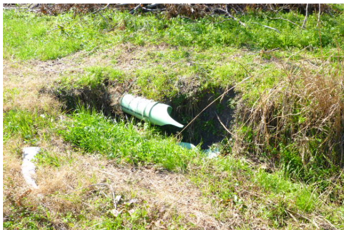
Figure 3-5: Example illicit discharge, Willow Springs Bayou
