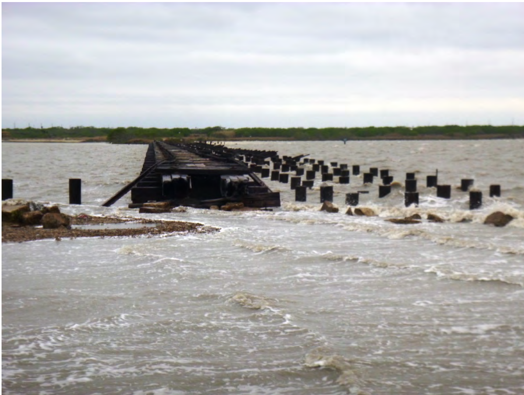
Figure 3.7. Access road submerged at Station 17119 during a storm at high tide.
