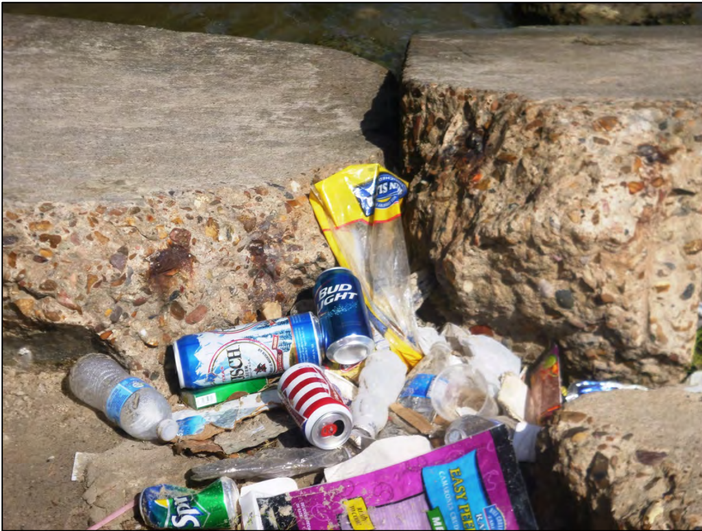
Figure 3.10. Station 13440 – Trash deposited among concrete riprap.
