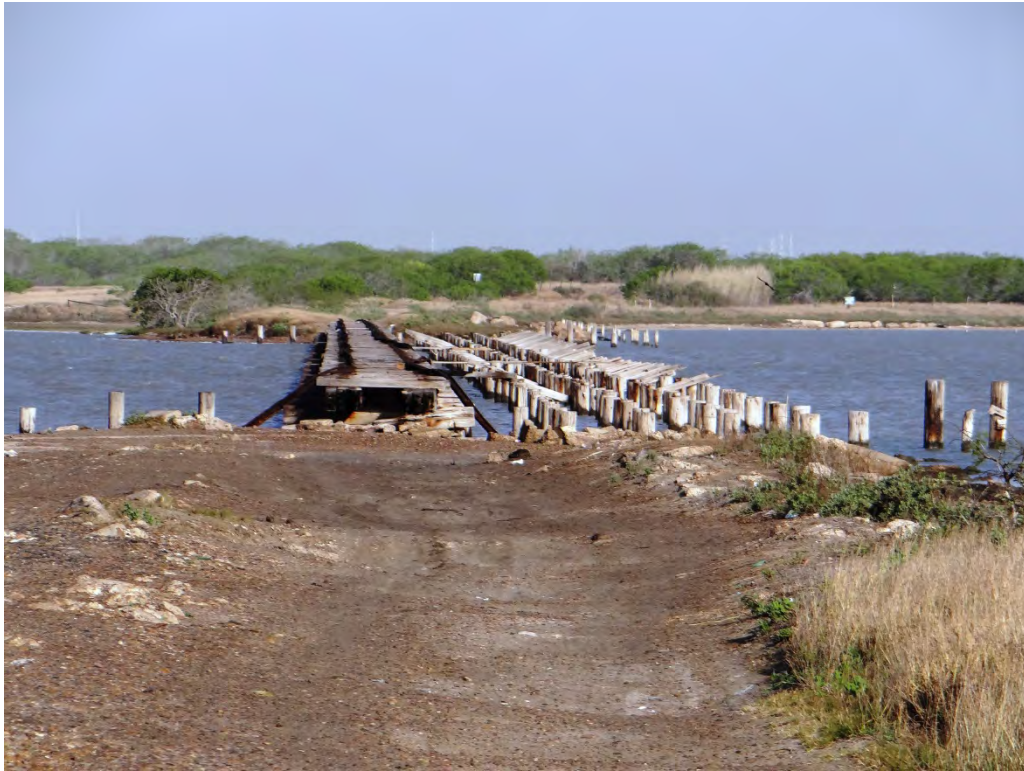
Figure 3.5. Station 17119 – Approach to station at the abandoned Holly Road Railroad tracks over Oso Bay.
