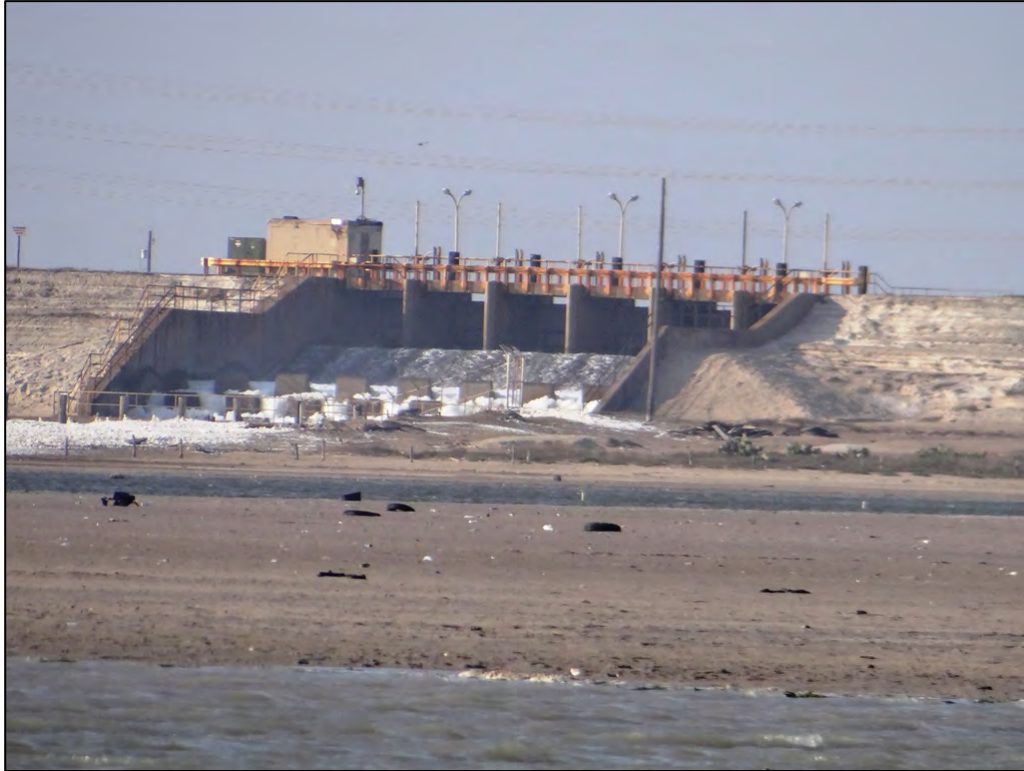
Figure 3.3. Cooling pond outfalls at the Topaz Energy Group-Barney Davis Energy Center.
