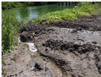
Runoff from bridge construction area observed entering Oso Creek
