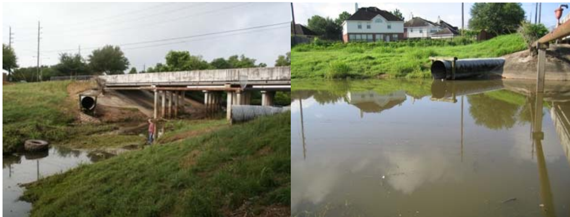
Figure 2-4 Photographs of Oyster Creek at Dulles Avenue a) normal conditions and b) during backwater event of July 2007
